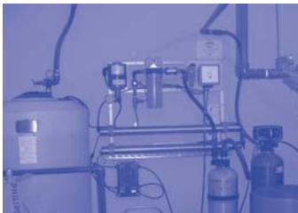
Efficient water treatment equipment can help reduce water consumption.
