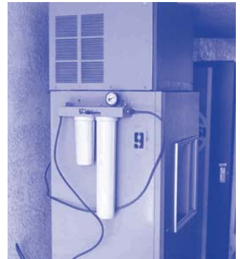
Air-cooled ice machines save water.
