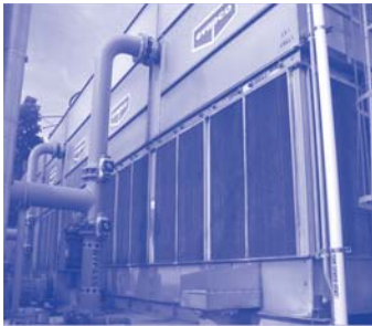
Typical cooling tower
