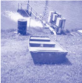
A pond at the Freescale plant in Oak Hill used to harvest stormwater for non-potable uses.
