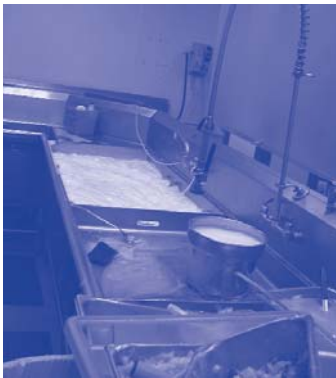
Typical pot and pan washing facility with power soaker
