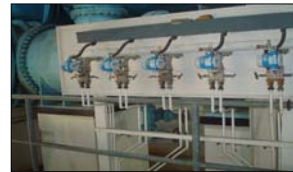
Bank of Differential Pressure Cells connected to flowmeters (Courtesy of Louisville Water Company)
